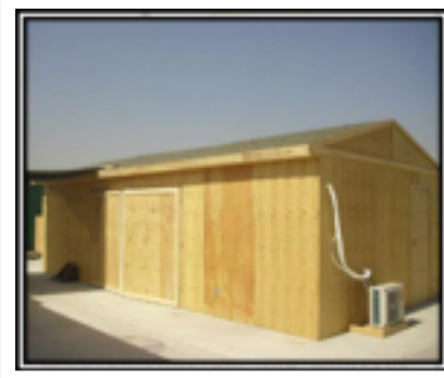
Build Team Two's modified B-hut structure completed for the Special Operations Forces
